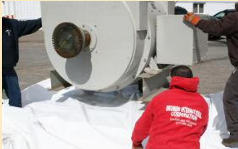
Left: A vapour barrier is laid over the platform base prior to the engine being lowered onto it.
